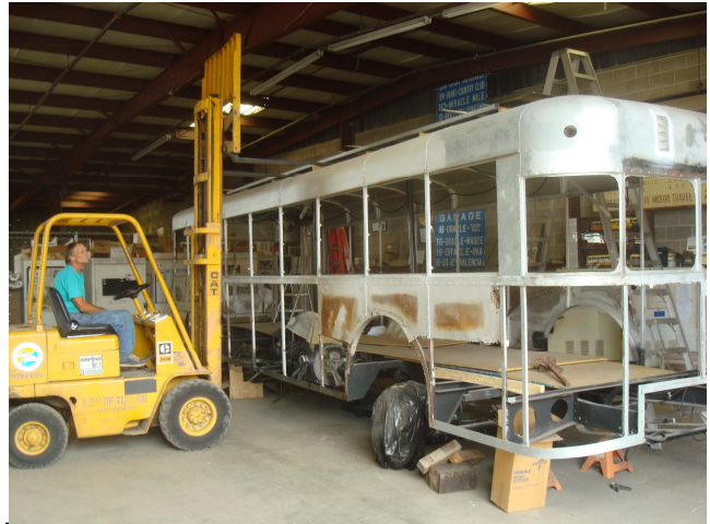
Dennis Gibbs on fork lift placing new center roof section on top of bus on June 2, 2012
