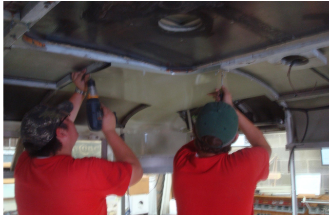
Student interns Alex Bauerelen and Tommy Ogden installing ceiling panels on July 26, 2013.
