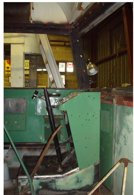
This photo shows the dash and adjacent wall panels mounted above the new driver’s platform flooring in September 2011
